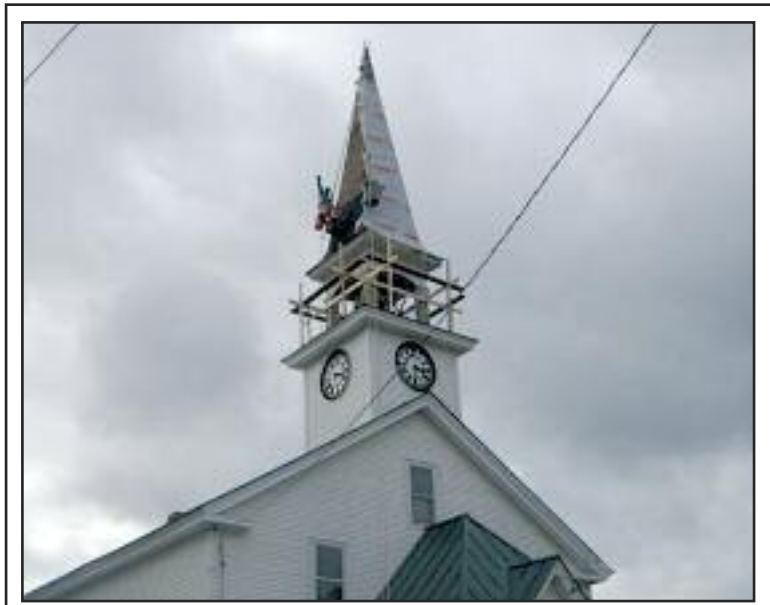
The Amazing Steeple Man. One member of the crew that is working on the steeple at the South Ryegate Presbyterian Church. The church continues to raise money for the restoration fund for that historic steeple. Photo by Carolyn Darling.
