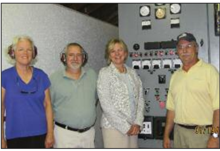
“Representative Suzanne Smith, Representative Paul Simard, and Senator Jeanie Forrester meet with Richard Mauser, who runs the hydro facility in Bristol. The legislators also toured another small-scale hydro facility in Campton. Both facilities are owned by members of the Granite State Hydropower Association (GSHA). There are 80 small-scale hydro facilities in New Hampshire.
